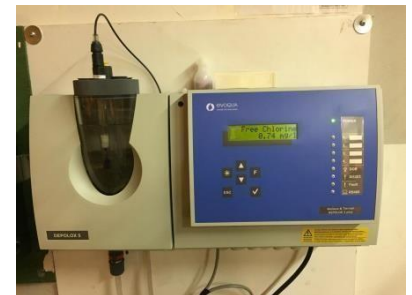
Online chlorine analyzer at Whalley Pump Station
