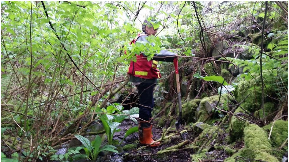
Photo 11. (WP19-2). Lyncean Creek East (179 Street culvert crossing). View of over-steepened rip rap slope at inlet culvert crossing
