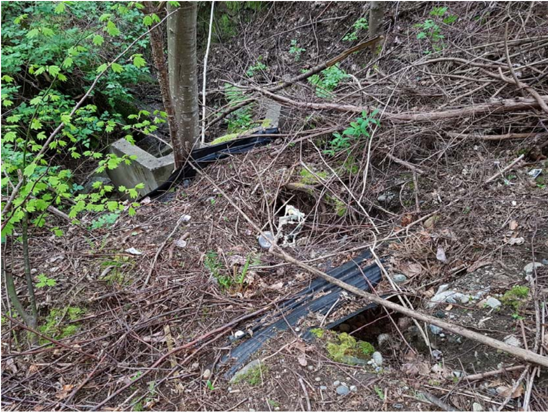
Photo 15. (WP18-4). Lyncean Creek West (West Tributary). Bank Erosion Above Culvert at 100 Ave & Lyncean Dr.
