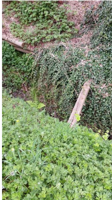
Photo 1. (WP-182A ST DITCH) 182A Street Ditch. View of left bank decaying and toppling landscape tie retaining walls and wall debris.
