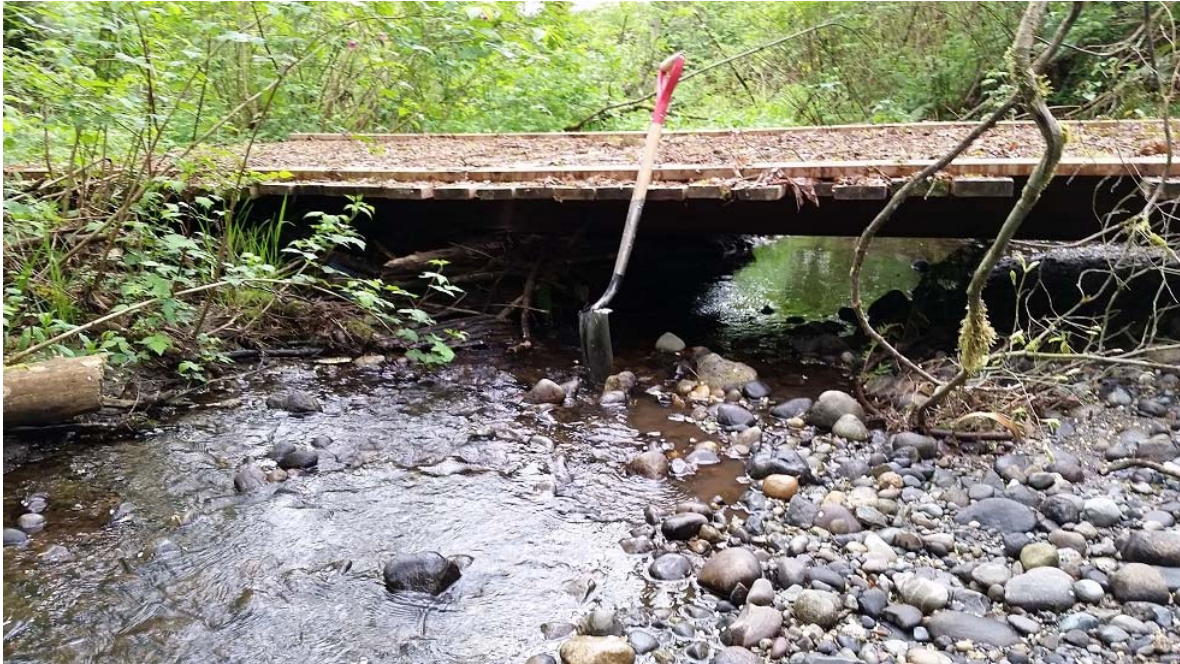
Photo 5. (WP20-BRIDGE). Leoran Brook (middle section). View of amateur footbridge crossing with woody debris accumulating under the bridge against the stringers.
