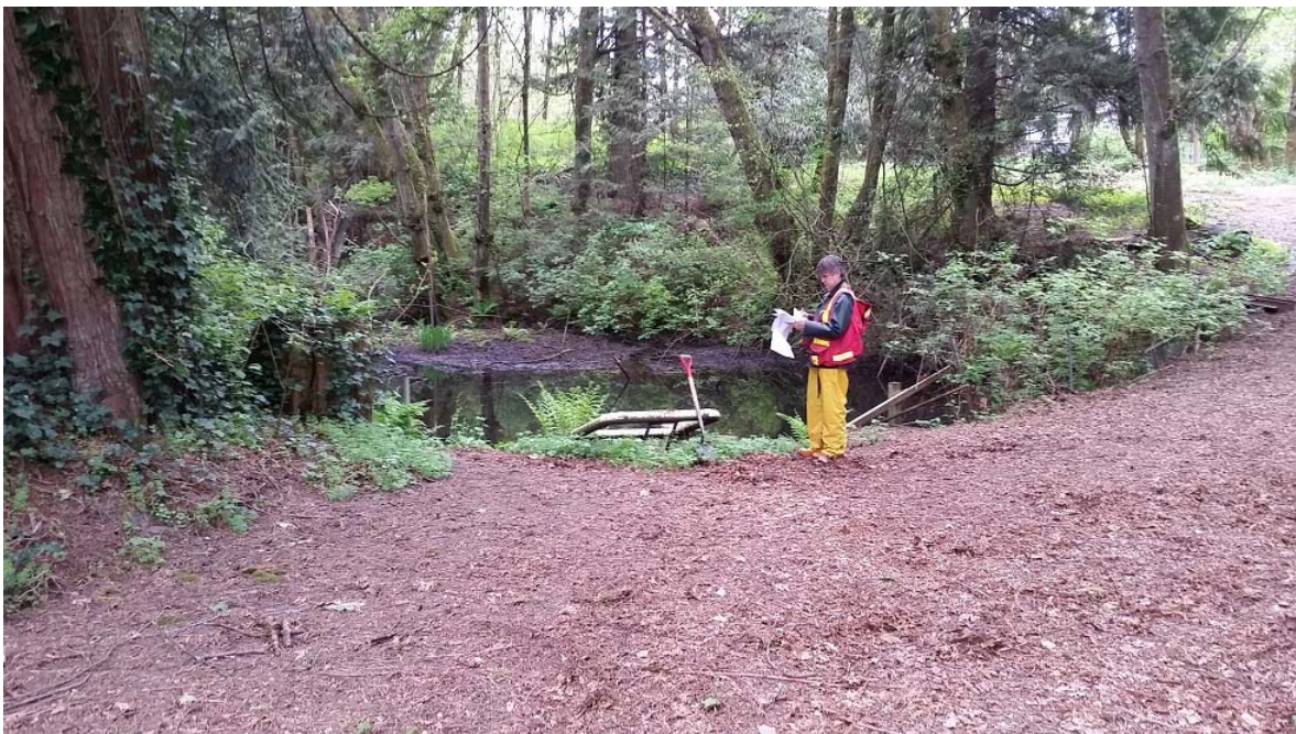
Photo 8. (WP19-14). Lyncean Creek East. View of upper pond (access road ravine fill). Culvert trash rack partially clogged with debris
