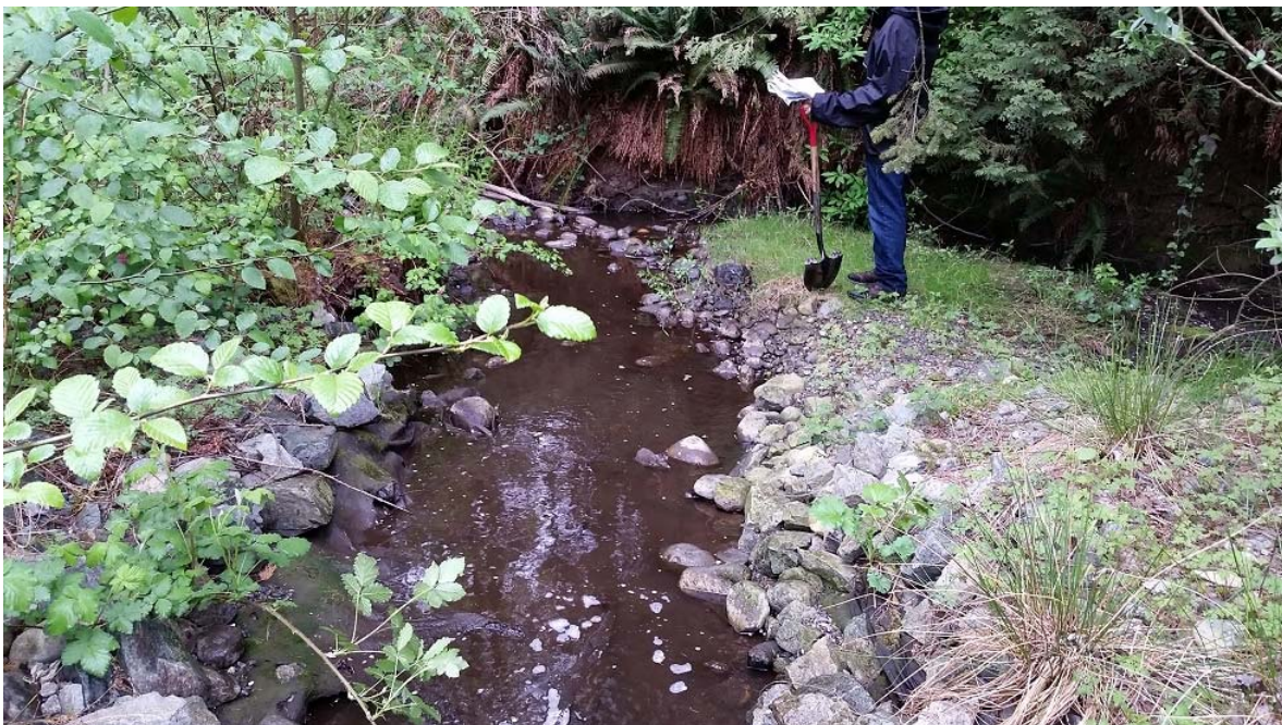
Photo 2. (WP20-1) Leoran Brook (upper section at Hwy 1). View of right bank erosion and recent instream works (~5 yrs old).
