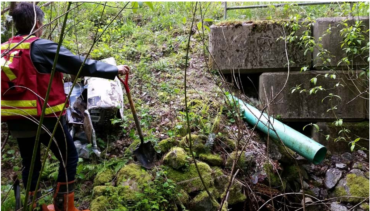
Photo 10 (WP19-2). Lyncean Creek East (179 Street culvert crossing). View of 200mm pipe draining northbound roadway scupper and Lock Block retaining wall erosion.
