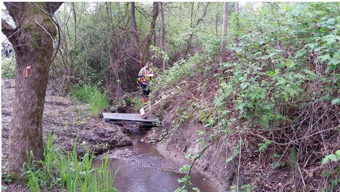
Photo 18. (WP18-SOLDIER PILES). Lyncean Creek West. View of right bank fill and near vertical (excavated) left bank slopes
