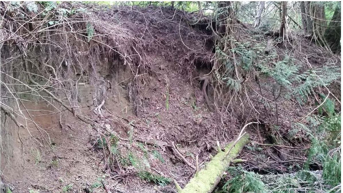
Photo 4. (WP20-EROSION) Leoran Brook (middle section). View of left bank erosion and woody debris
