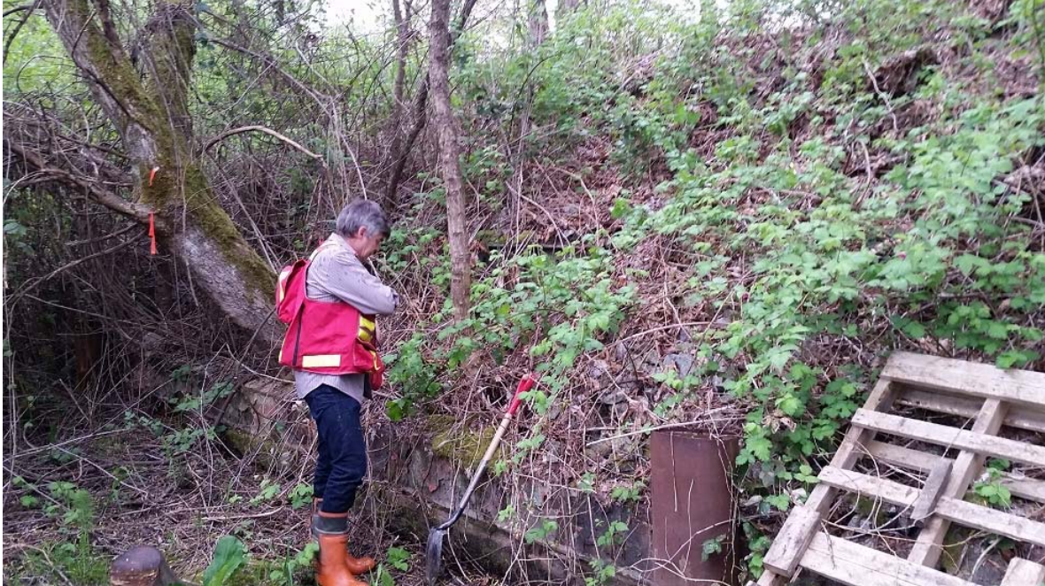
Photo 17. (WP18-SOLDIER PILES). Lyncean Creek West. View of left bank tiered soldierpile walls (~300mm steel pipe piles with various metal lagging).
