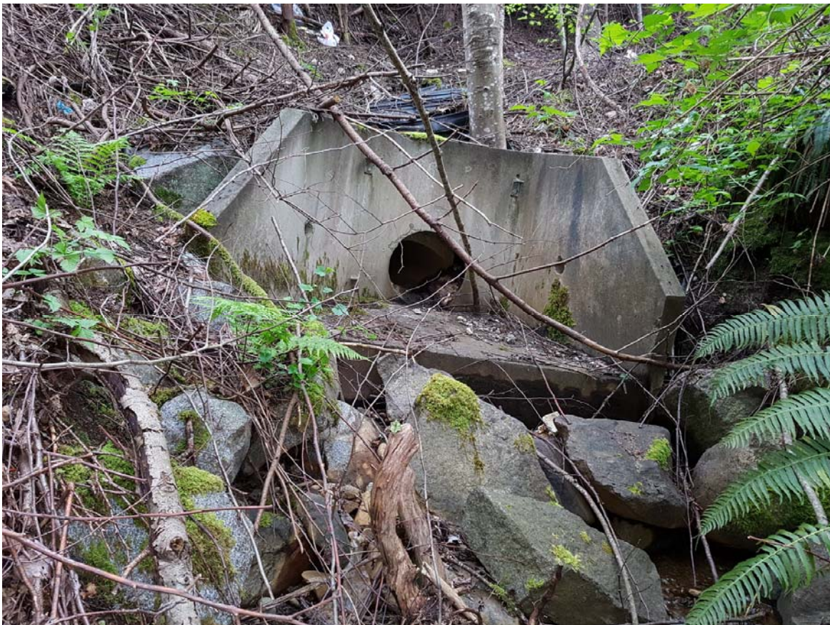
Photo 14. (WP18-4). Lyncean Creek West (West Tributary). Undermined Culvert Headwall at 100 Ave & Lyncean Drive.
