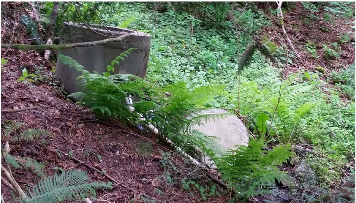
Photo 12. (WP18-FILL/SUMP). Lyncean Creek West (East Tributary). Small scale stormwater control structure (vandalized) flowing approximately 5gpm.
