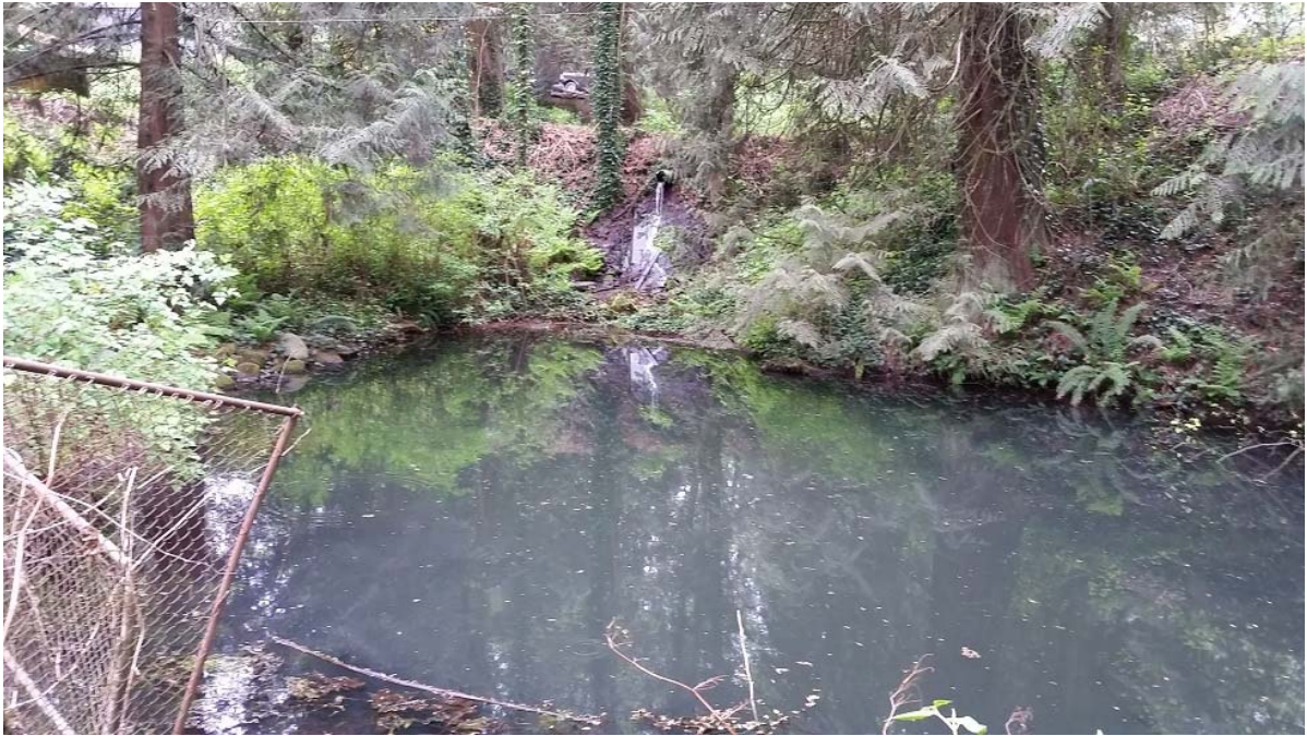
Photo 9 (WP19-14). Lyncean Creek East. View of main pond showing flow from upper pond through access road ravine fill. Main pond trash rack damaged and partially clogged with debris.
