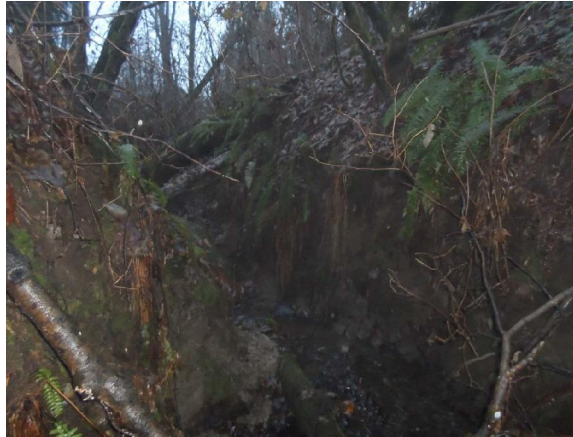
Photo 21: Unstable banks of headwater stream near 179 St.
