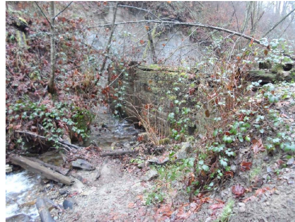
Photo 10: Old wooden water supply dam and slope failure on left bank
