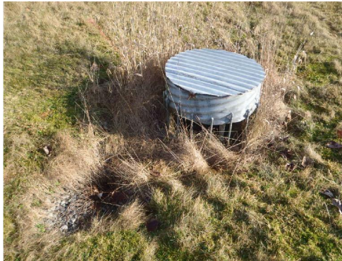
Photograph 5 Rock drain at bottom of dispersal pit, 158 St.
