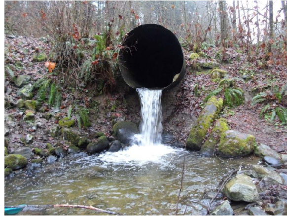
Photo 9: Hanging CV (fish barrier) on Bon Accord Creek at trail crossing
