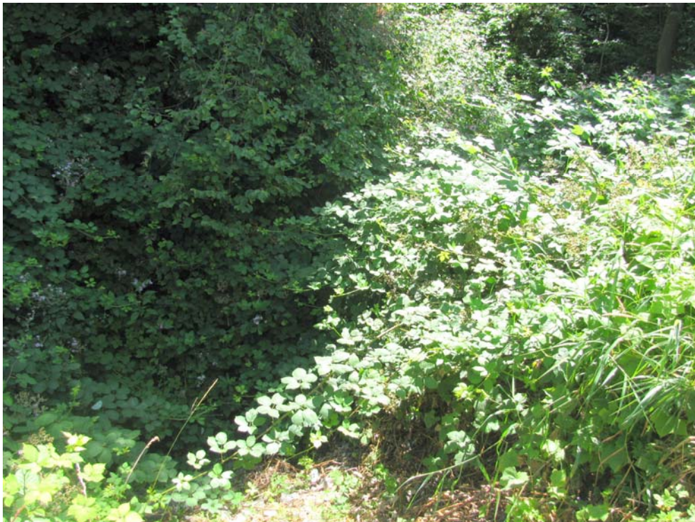
Creek 274 at 184 th Street, ravine condition adjacent to road (view east)
