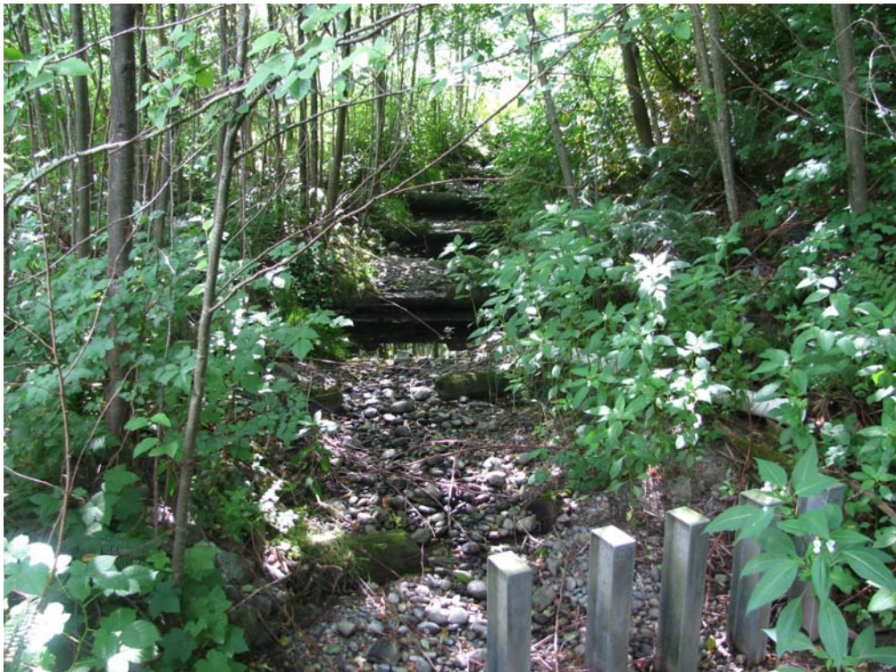
193 rd Street Creek at 80 th Avenue (view upstream, grade control and trash rack)
