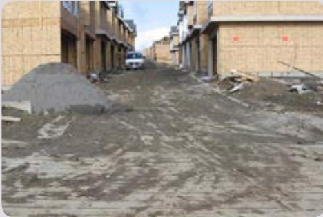
The above demonstrates inappropriate stockpile handling, and dirt accumulated on the road from construction sites with no BMP's. The accumulated dirt is then tracked further by site traffic.
