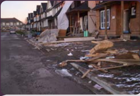
This single family construction site shows no ESC management on-site. Perimeter controls, surface protection, a gravel access pad and regular road sweeping should be implemented to prevent stormwater pollution.
