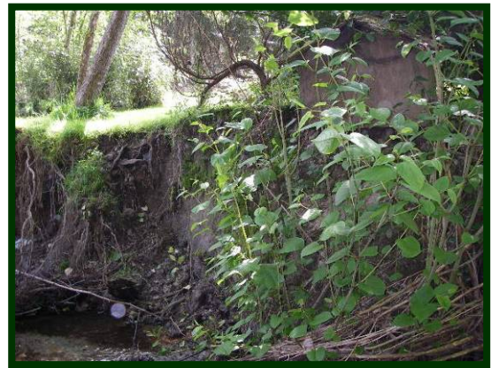
Photo 7.2: Erosion in Hyland Creek near Site H2
