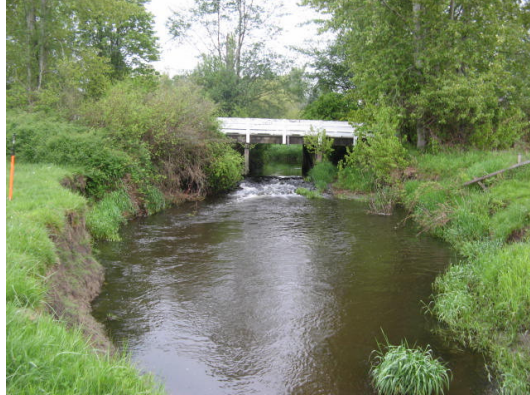
12 Avenue Bridge & Erosion
