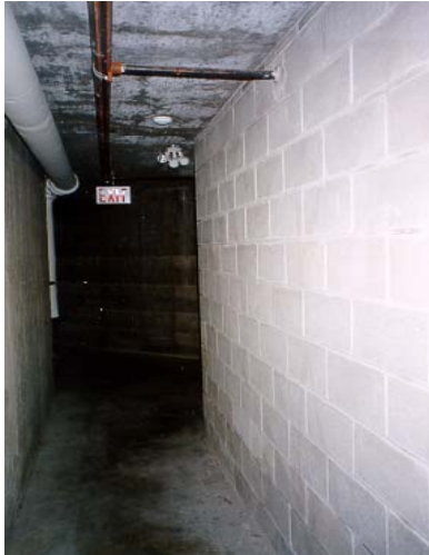
Poorly lit corridor with no surveillance.
