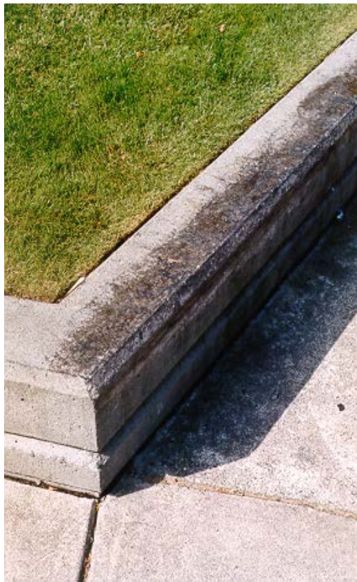
Skateboard damage to concrete curb.
