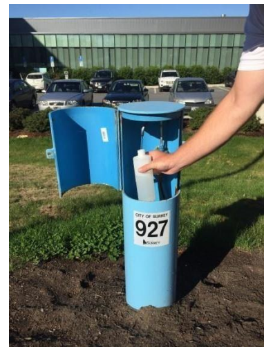
Water Sampling Station at 148 St.
