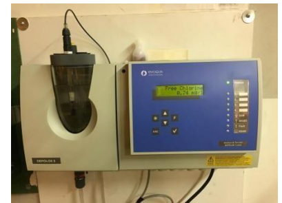
Online chlorine analyzer at Whalley Pump Station
