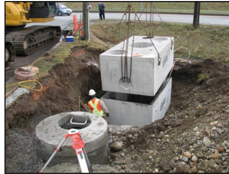
Oil Grit Separator
