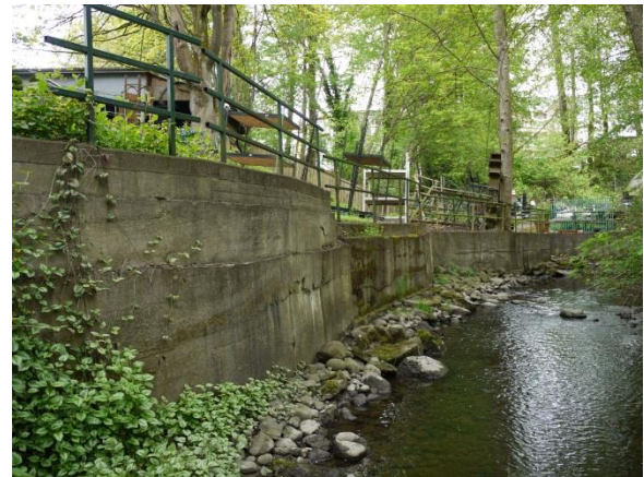
Photo 4-2: Some encroachment from residential development and invasive species issues
