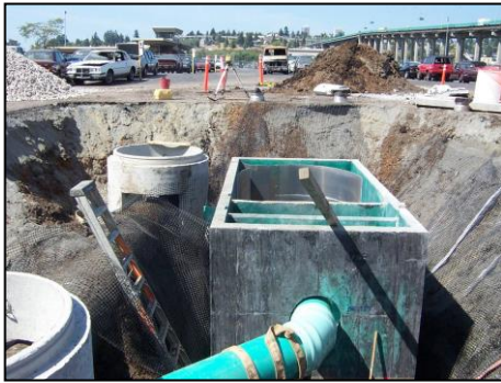
Oil Grit Separator
