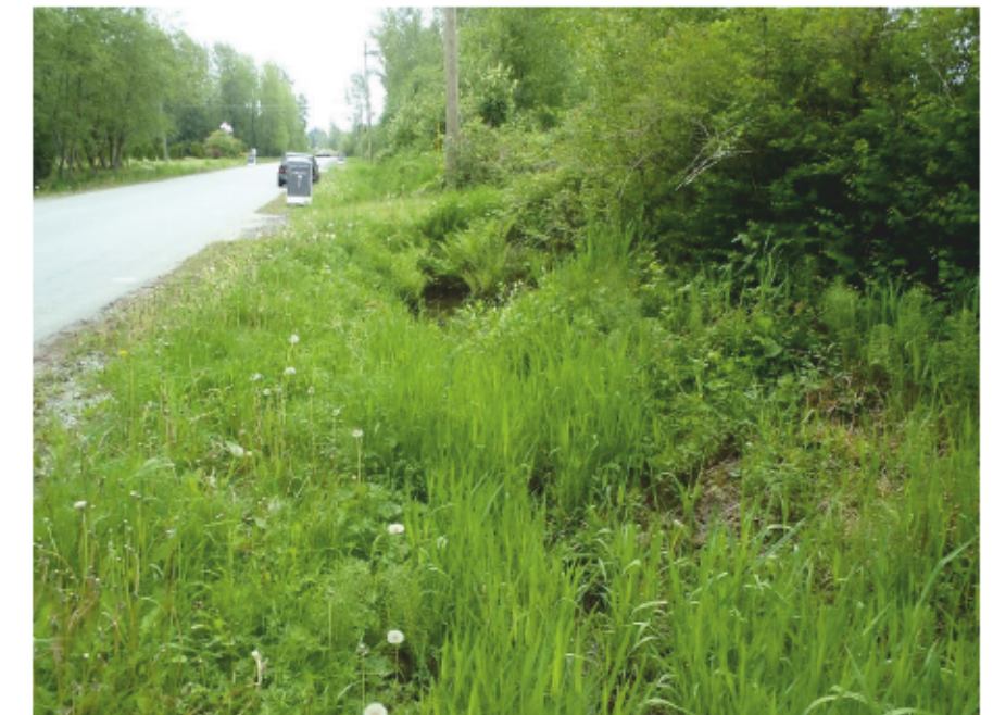
Photo X: DS (south) view of roadside ditch along the west side of 172 St., south of 16 Ave.
