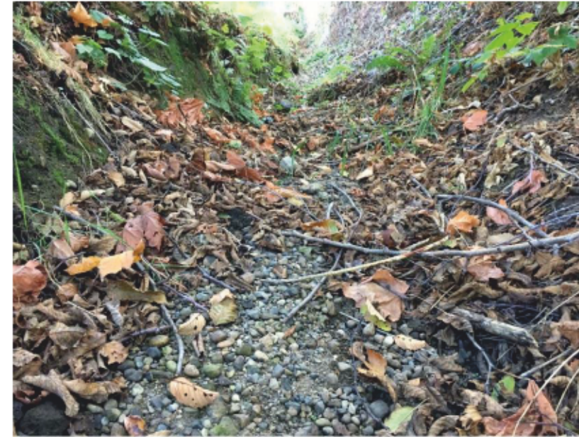
Photo 14: Class B Watercourse. Downstream view of Watercourse 3 from mid-channel with gravel substrate.
