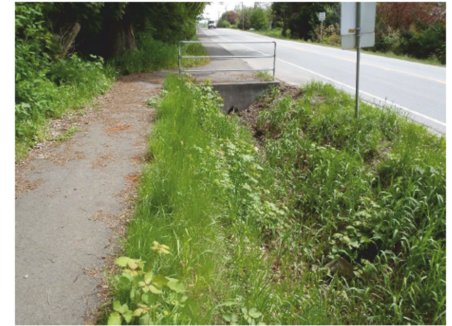
Photo U: DS (east) view of roadside ditch along north side of 16 Ave., east of 172 St.
