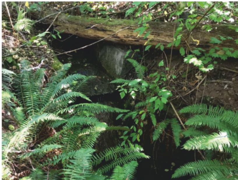
Photo 19: Class B Watercourse. Upstream view of natural barrier with concrete flume in Watercourse 5 approximately 100 m upstream from 18 Avenue.
