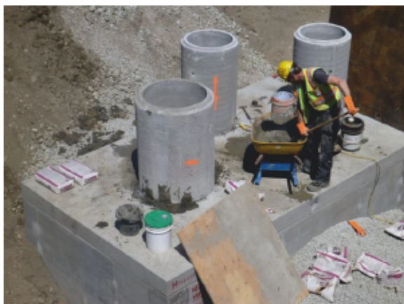
Structural Treatment Device
