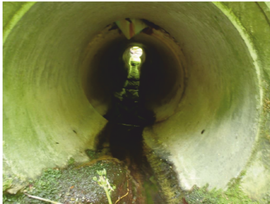
Photo Q: DS (south) view of concrete culvert at 16 Ave., east of 172 St.
