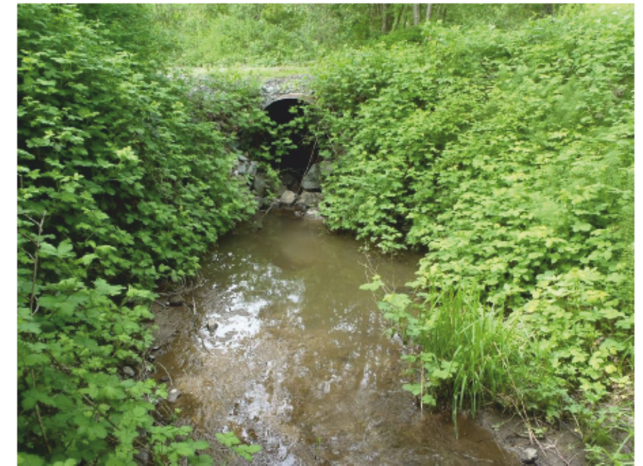
Photo AD: US (northwest) view of Sam Hill Creek and perched culvert between 172 St. and 176 St.
