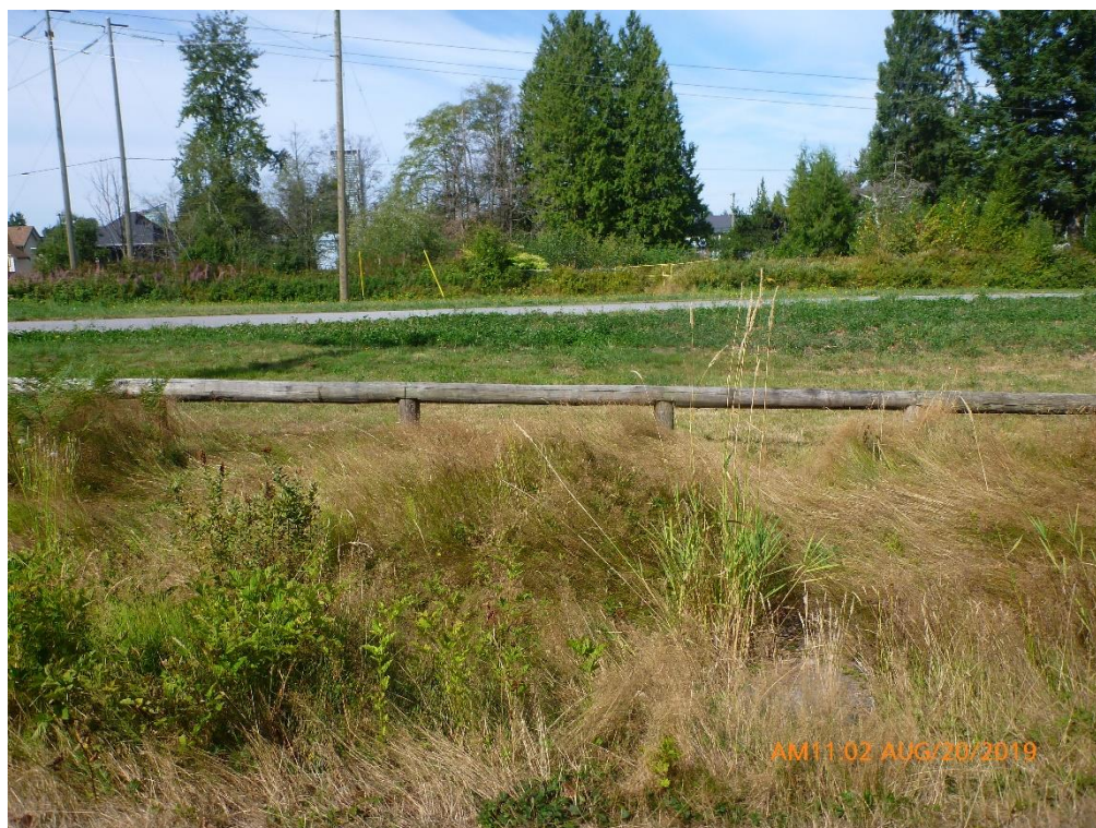
Photo 9. Class D ditch across from lot 10492, left bank (west) view. The site is pictured in the background.
