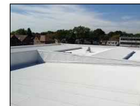
7 SOPREMA SPOPRASTAR HIGH ALBEDO ROOF WITH SRI VALUE OF .82
