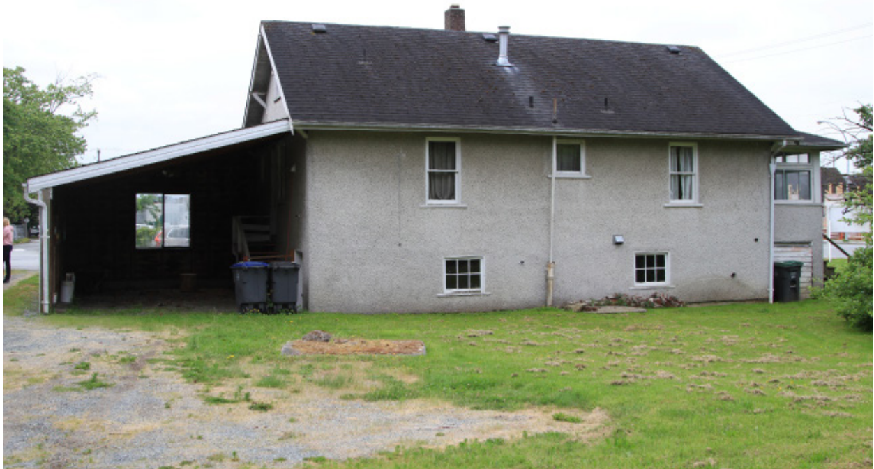
Side (north) elevation of Main Residence, showing later shed-roof extension to the rear (left) and front verandah (right). Note uniform settlement at northwest corner of front verandah.
