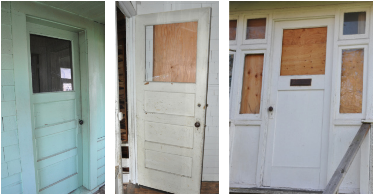
Photos showing typical primary and secondary exterior doors: Note that the primary (left) and secondary (middle) entry doors inside the front verandah and rear porch are characterized by a glazed upper and three wood lower inset panelling. The existing closed configuration of the front verandah appears to be an early alteration, which features a ribbon of wood window sashes with corresponding transom band above in the same width, and an in-swing door sash (glazed upper and wood lower inset panelling) with paired sidelights.
