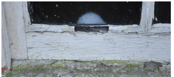
Photo showing typical deterioration of existing wood sashes.
