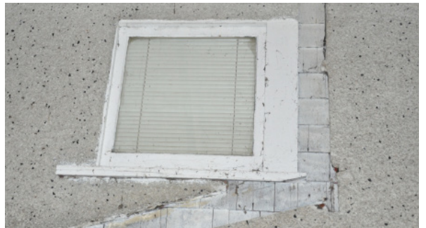
Fixed wood window at rear (east) elevation). Note exposed original wood window exterior casing, which would have been a typical trim detail for all window openings.
