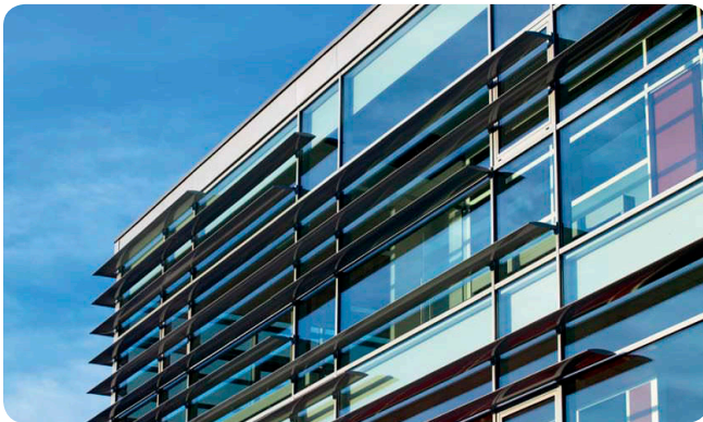
Horizontal shading devices can be added to a building's south and east facades where balconies are absent, or where they do not provide adequate summer shading.
