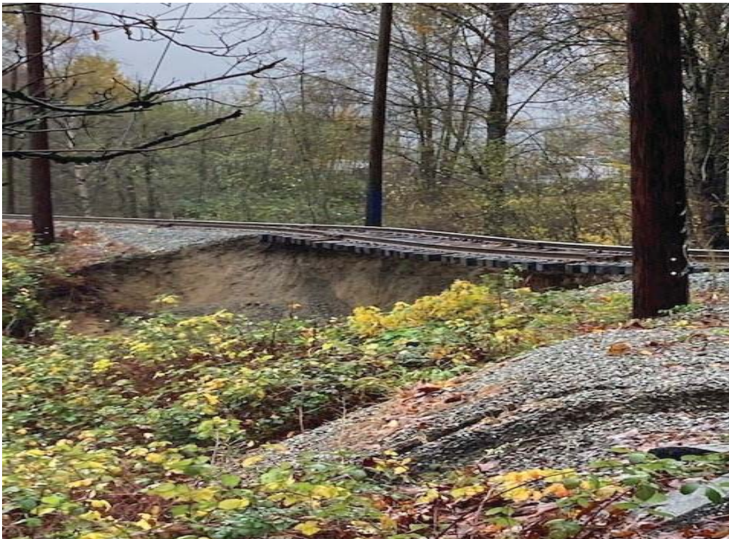
Bank Failure near Old Yale Rd and 125A St; Looking North on Old Yale Rd
