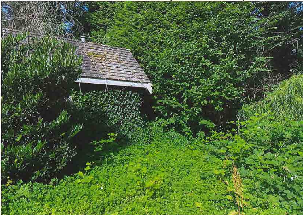
Photo 2: Outbuilding and unmaintained front yard with invasive species.
