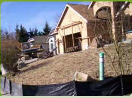
All sites large and small are expected to ensure that BMPs are implemented on the construction site, like the ones shown on this home building project.
