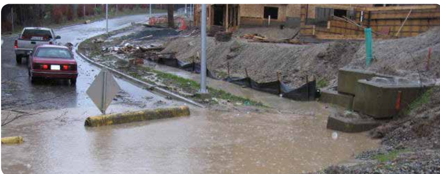
ESC Permits aim to ensure that occurrences like the one in this picture are prevented through appropriate site planning and management.
