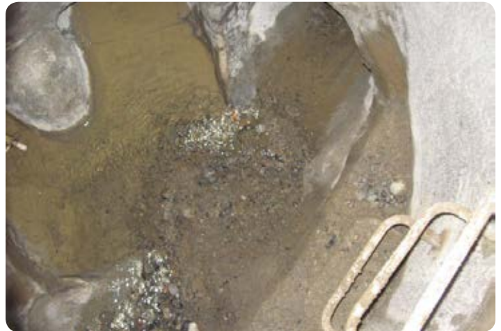
This image shows sediment that is beginning to accumulate in the pipe system.
