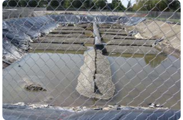
The sediment control facility pictured above is an example of one of the many BMP's that may be specified by the Engineer to manage the stormwater pollution by sediment, from the construction area.
