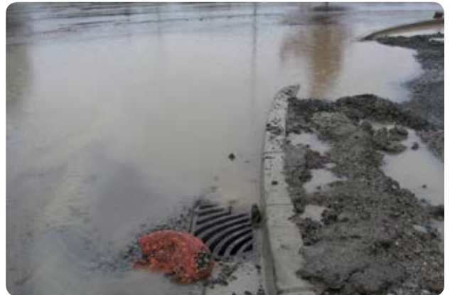
Many deficiencies become obvious during rainfall, regular site inspections ensure that such issues are identified and that action is taken to manage similar occurrences in the future.
