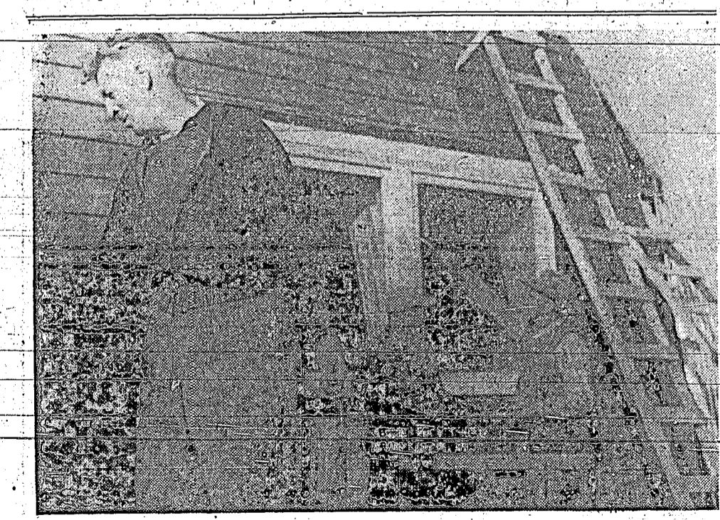
Busy with paint pot and brush are these members of the Valley Curling Rink, who are helping to build the 6-sheet ice rink on the Fair Grounds, Cloverdale.
