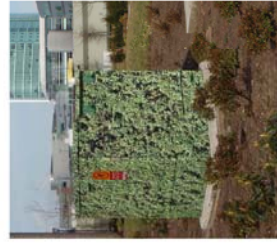
5. VINTL IMAGE INSOAP ON PINT HEDGE IMAGE; MUST BE APPROVED BY AND COORDINATED WITH BC HYDRO
