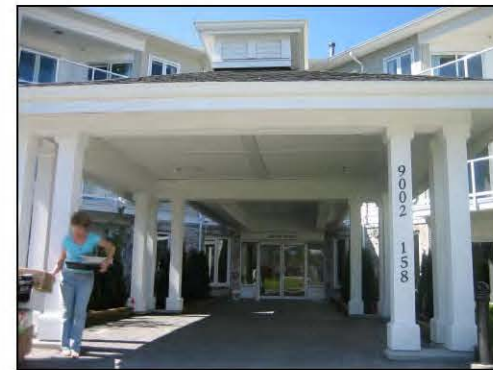
View of Existing Porte Cochere, Wood Clad Columns, White Trim and White Aluminum Entry Screens
