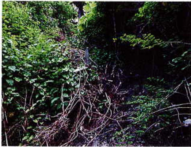
Photo No.05: evidence of past surficial slump Evidence of past surficial failure with surface erosion occurring located midway up the slope
