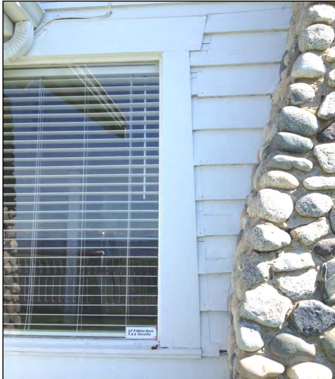
Photo 16: Window detail showing original trim design repeated for altered opening for contemporary direct-glazed window. Note line of original trims.
