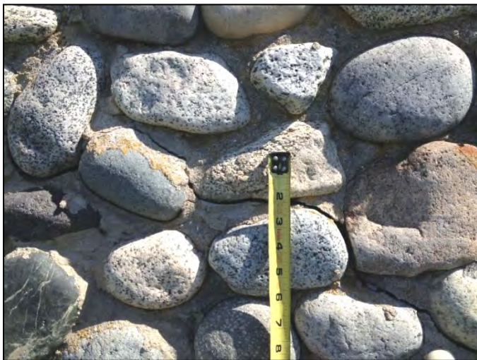
Photo 14: Typ. cracking of later mortar repairs.
