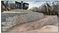
LARGE GRAVITY WALL BLOCKS, MAGNUM STONE. REFER TO GEOTECHNICAL ENGINEERING DRAWINGS & SPECIFICATIONS
