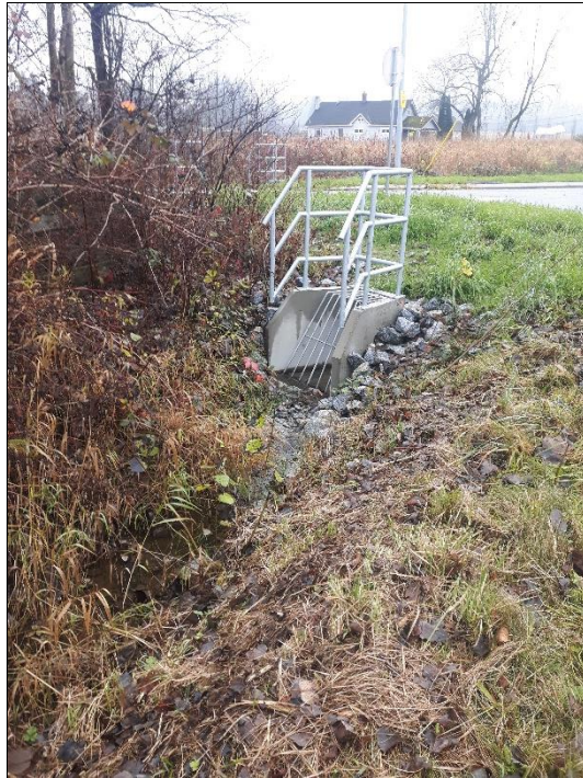
Photograph 3: 192 nd St. Ditch at intersection of 192 nd St. & 48 th Ave.
