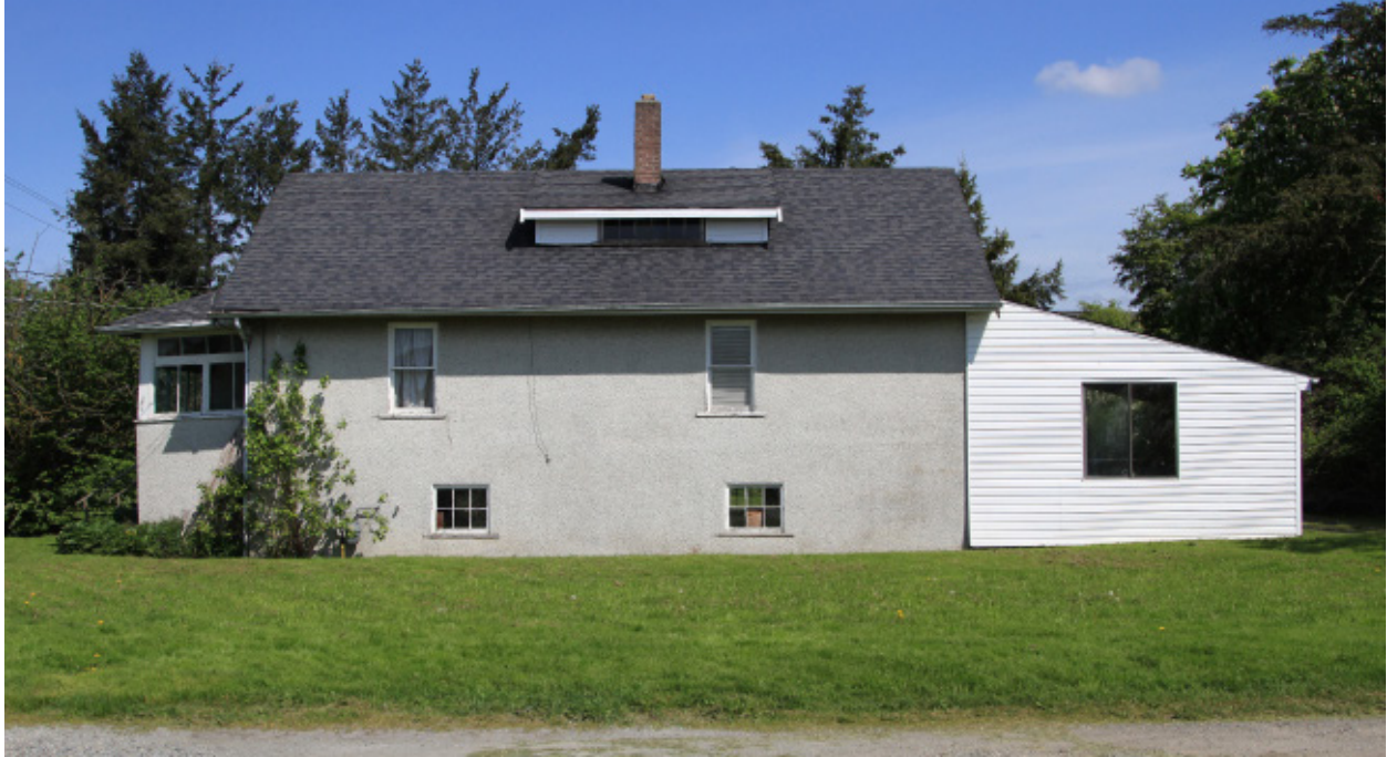
Side (south) elevation of Main Residence, showing front verandah (left) and later shed-roof extension to the rear (right). Note differential settlement at southwest corner of front verandah.
