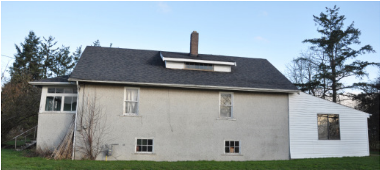
South elevation showing primary front-gabled wood-frame roof structure, shed dormer, interior brick chimney, hipped-roof (verandah), and shed-roof (rear extension, not original).
