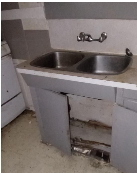
Figure 93: Rotten floor under kitchen sink
