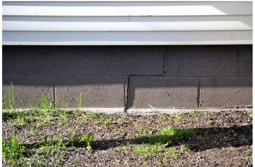
Figure 19: Disjointed concrete block
