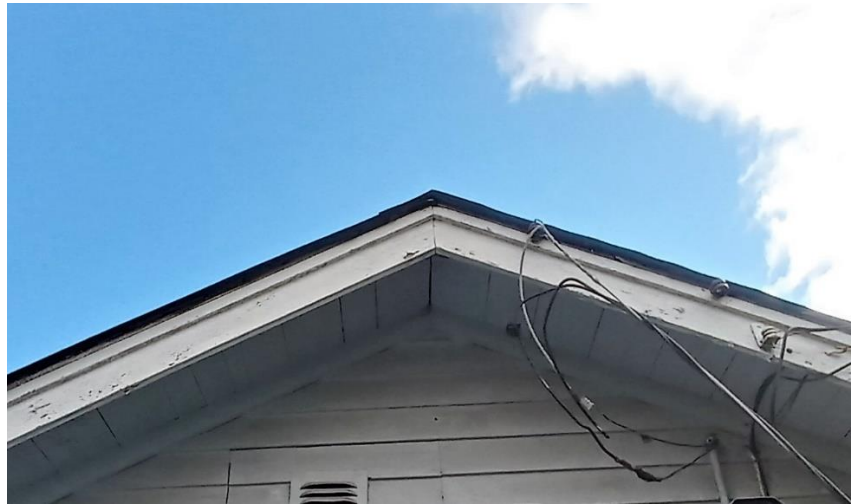
Figure 72: Exposed underside of roof decking
