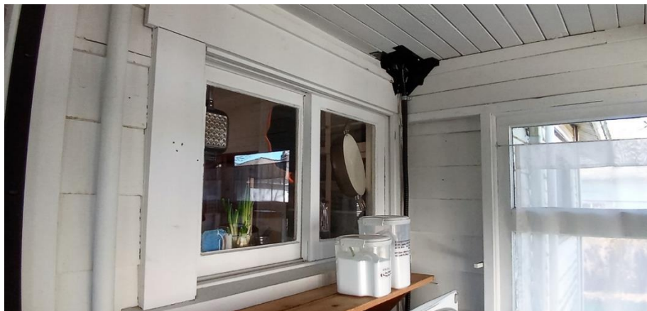
Figure 32: Interior of back porch with kitchen window on the left and cedar shingles on the wall
