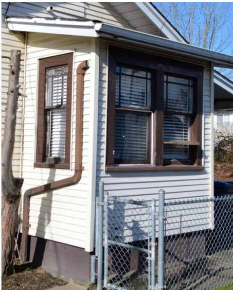
Figure 22: Disconnected eaves trough at dining nook
